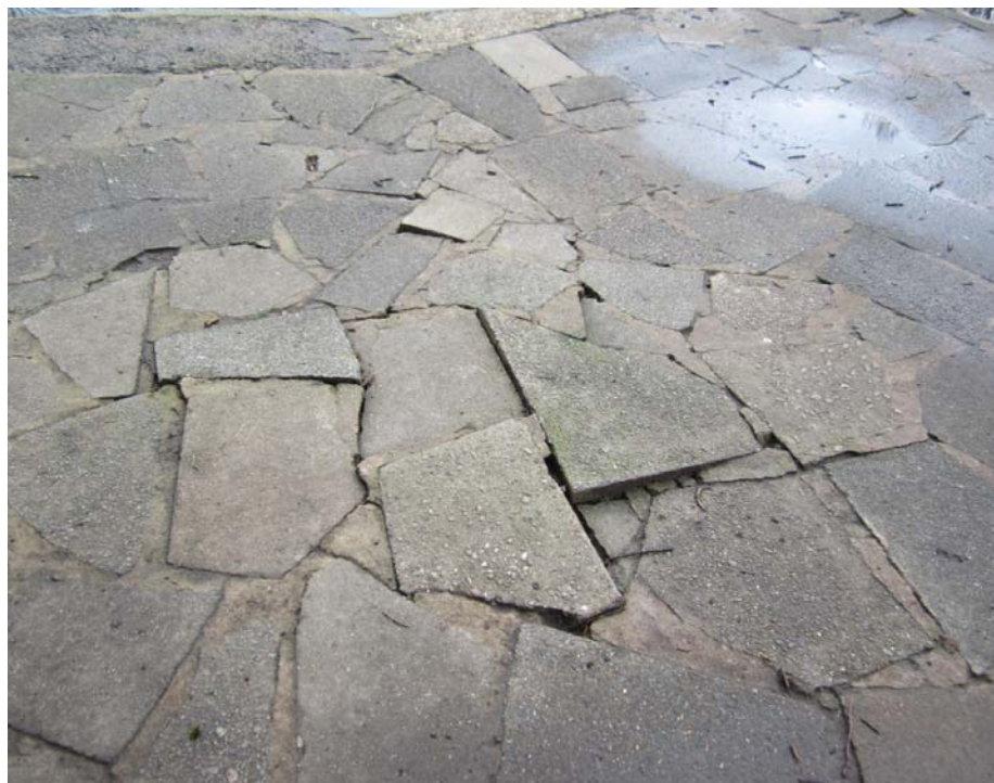
Hazardous crazy paving in need of repair
