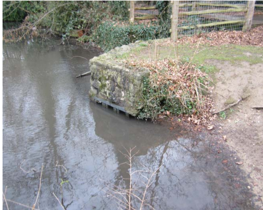
Eroded lake banks in central lake
