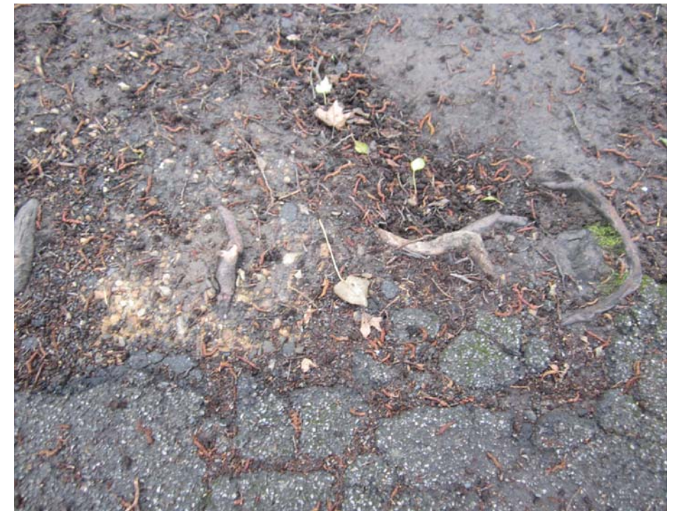
Damage to macadam due to tree roots
