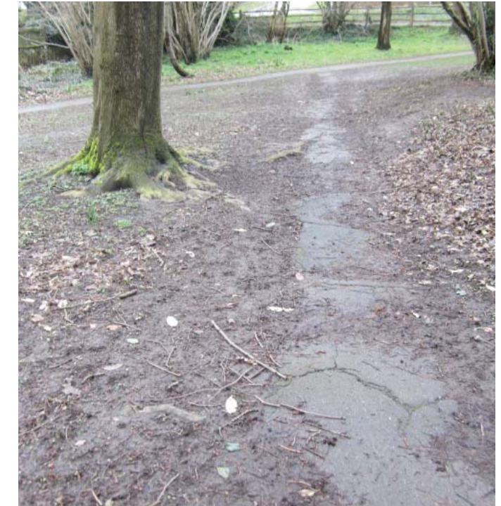
Macadam paths disintegrating
