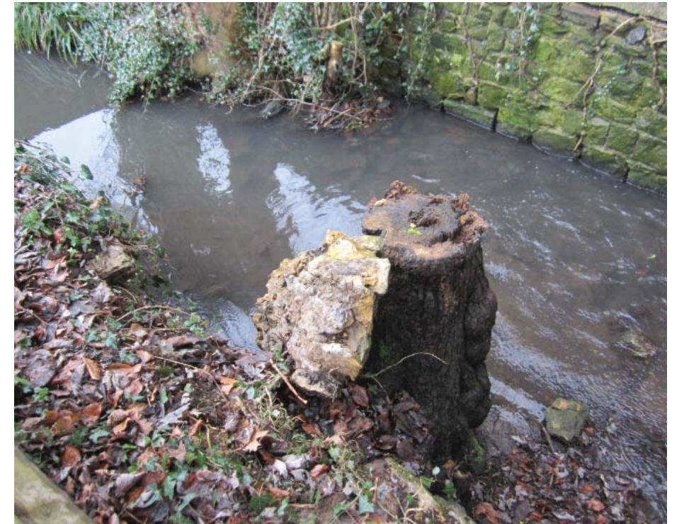
Collapsed stream wall
