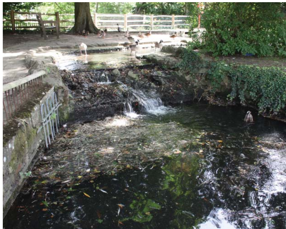
Waterfall wall in need of repair
