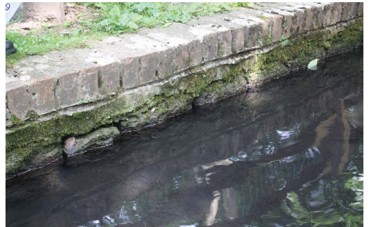
Repairs to stonework required
